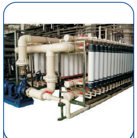
Ultra Filtration System
