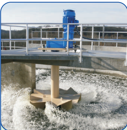
Fixed Surface Aerator
